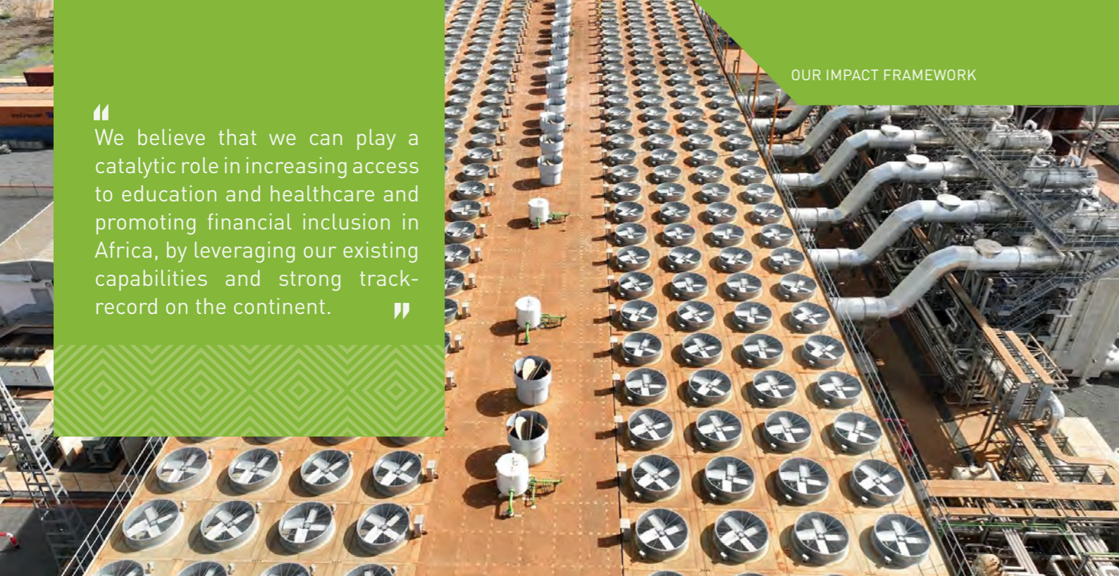
◆ Completed Malicounda Power Plant, Senegal
