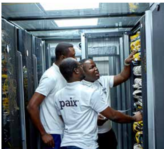
PAIX Data Centres: the Pan-African provider has operating data centres in Ghana and Kenya and has ongoing projects across the region
