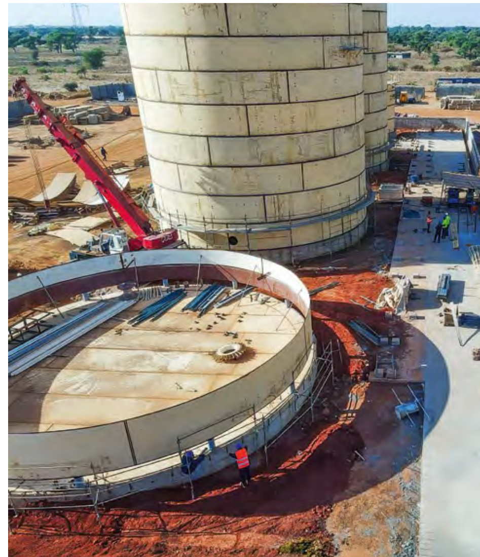
📍 Malicounda Power Plant, Senegal
