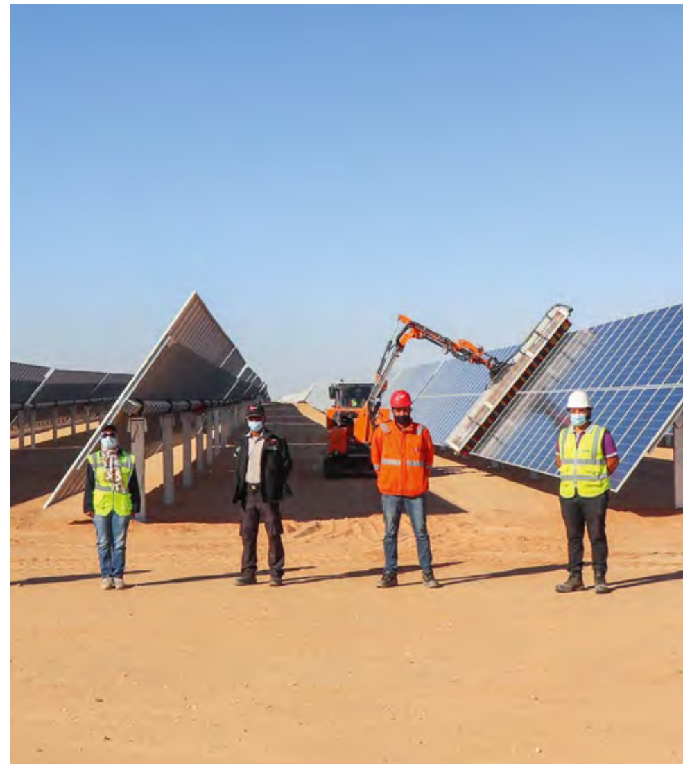
➤ Benban Solar Park, Egypt
