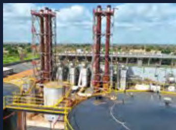
📍 Malicounda Power Plant, Senegal
