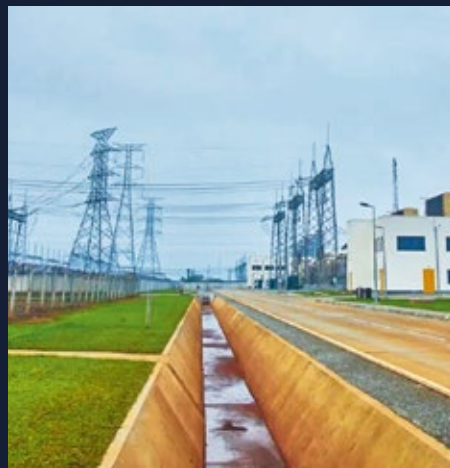
📍 Azura Edo Power Station, Nigeria
