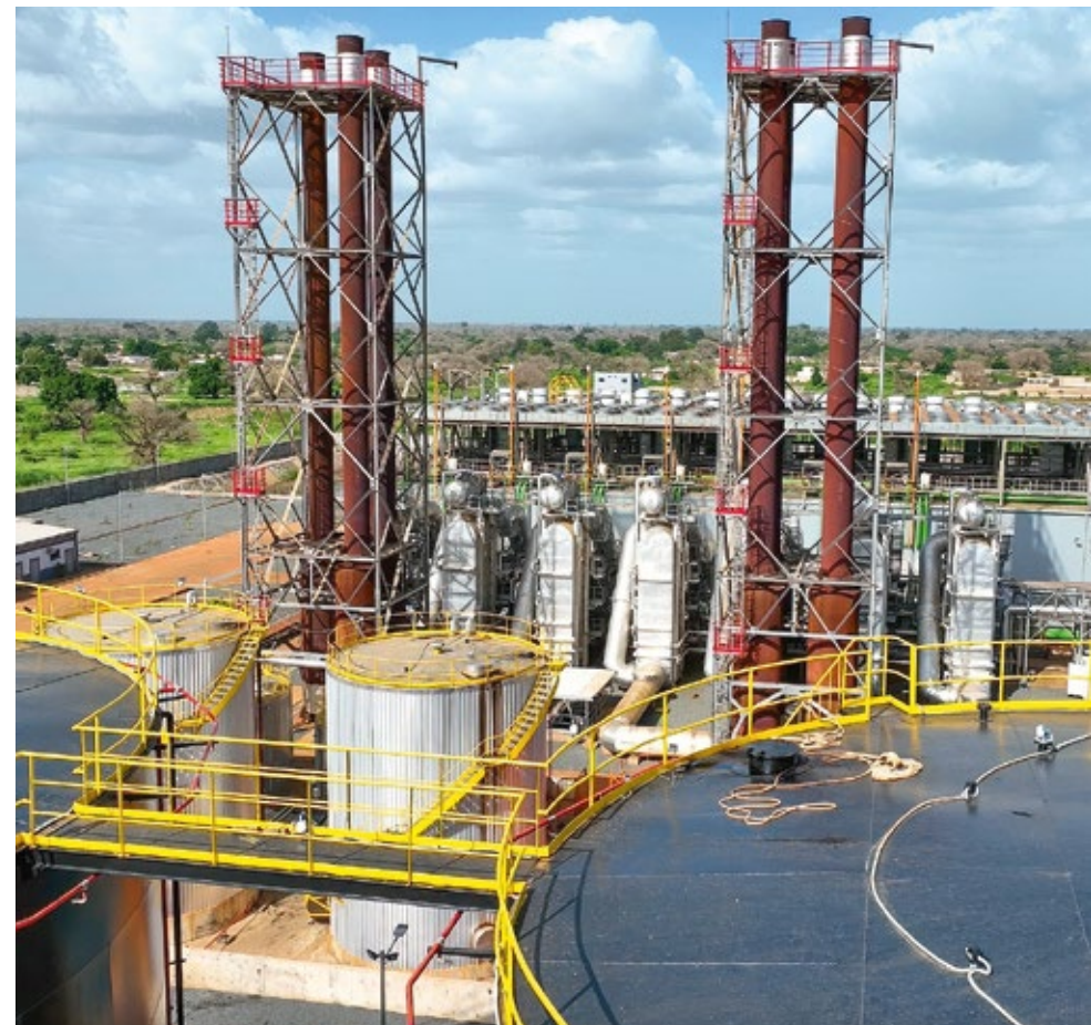
📍 Malicounda Power Plant, Senegal
